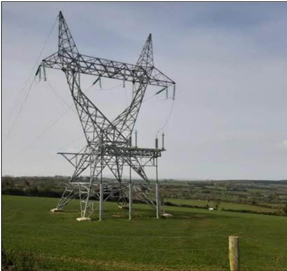
Figure 5-29: Photo of 220 kV Line Cable Interface Mast with shield-wire facility.
