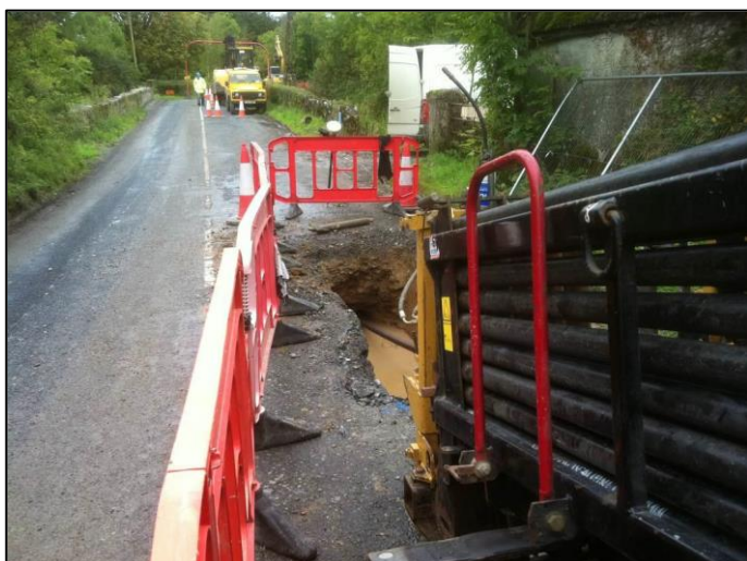
Figure 5-26: Standard HDD site on local road where HDD was used to go underneath a bridge (bridge parapet walls visible).
