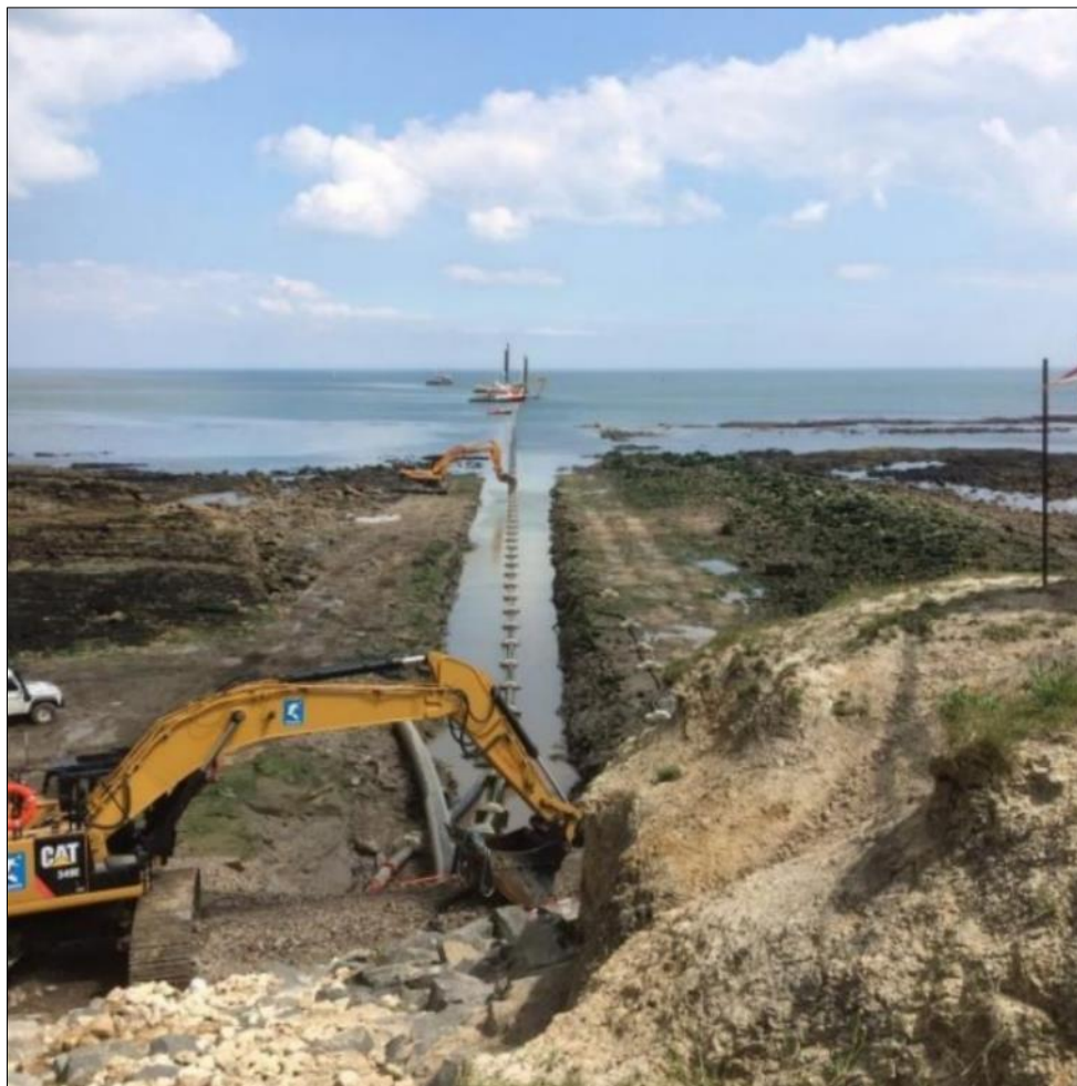
Figure 5-13: Photo showing installation of a cable in a trench at a landfall.
